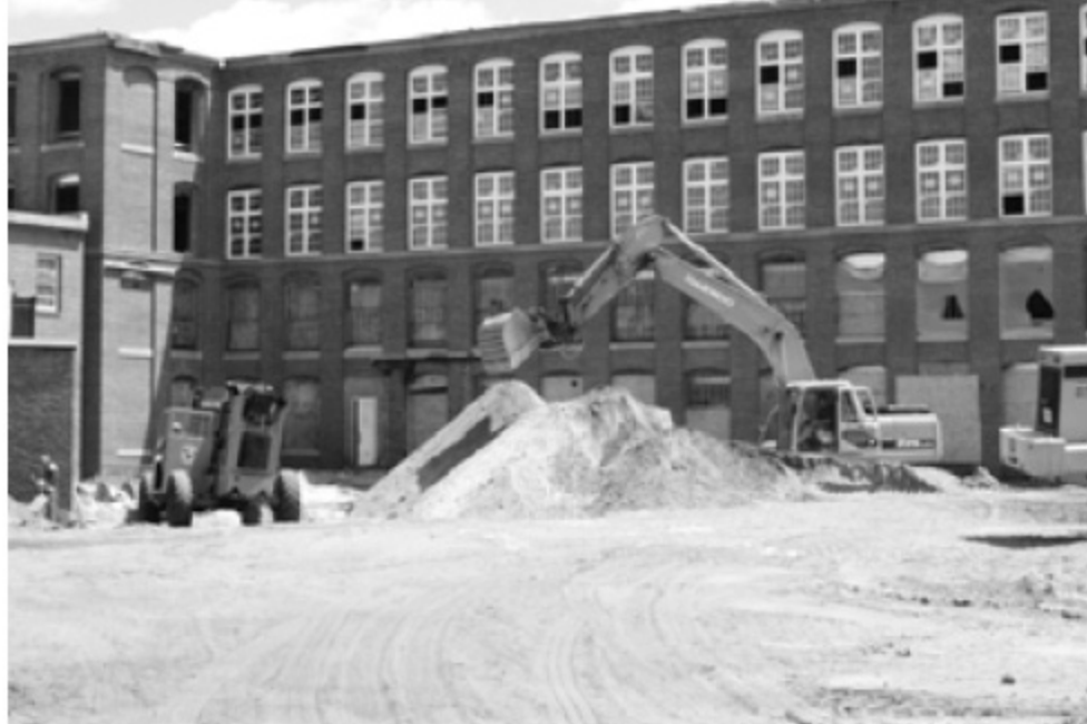
Renovations at the Silver Street mill complex are nearly halfway complete. (Express Photo/Dan Magazu)
